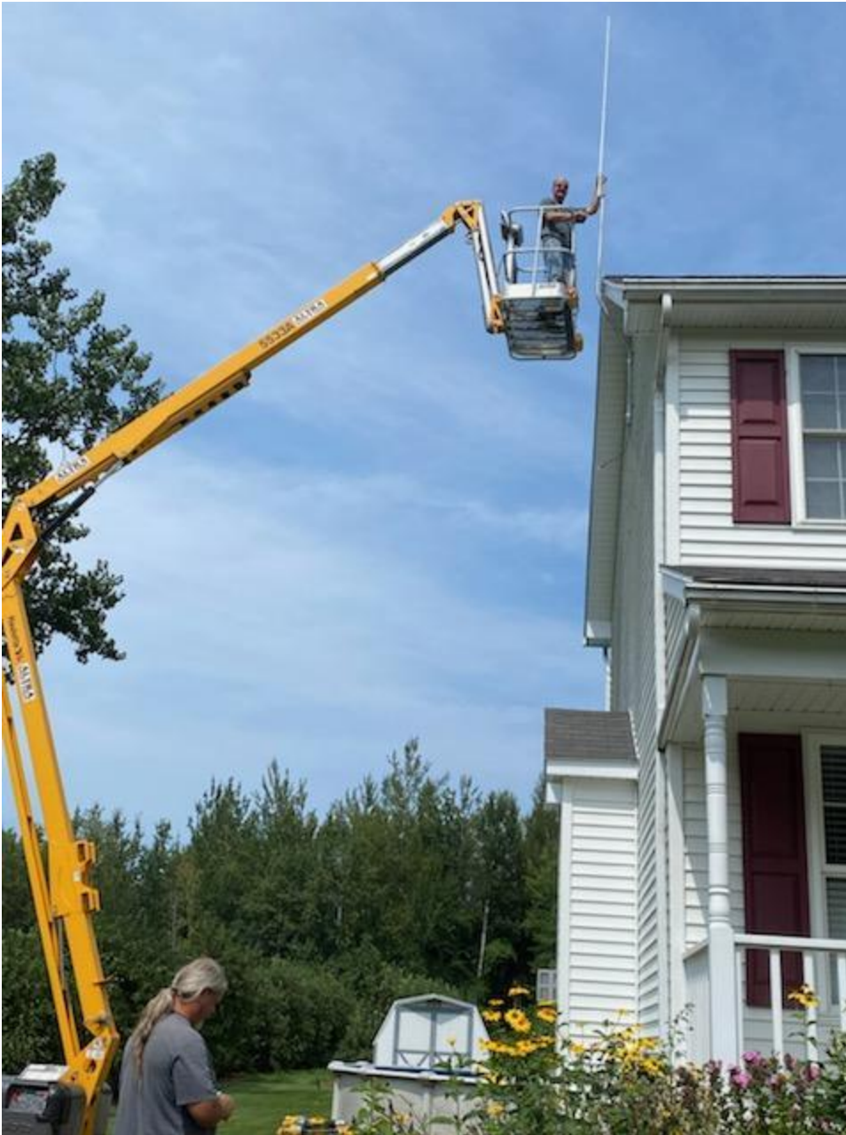
Dual Band Antenna installation by Dave KD2VNV. Nice and Safe, Dave!! Have fun.
